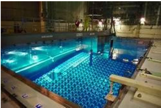
Spent fuel pool. Courtesy of RADēCO.
